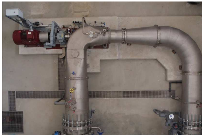
Figure 26 : Poggio Cuculo turbine (Italy) designed from Mhylab's systemization set within a drinking water treatment plant ( Q_n = 0.38 \text{ m}^3/\text{s} , H_n = 12.5 \text{ m} , P_m = 42 \text{ kW} , variable speed) (© Mhylab)
